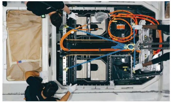
Candela boats sport Polestar batteries - could a lower-price option, featuring second-life energy storage, represent a viable solution for the future?
