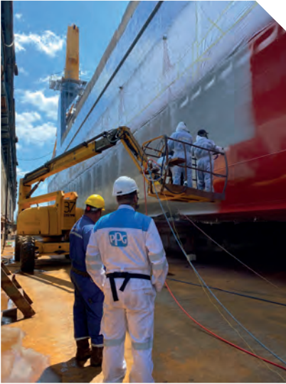
PPG SigmaPrime is applied as a base coat, followed by PPG SigmaGlide 790 as a tie coat, and finally the SigmaGlide 2390 as the top coat
